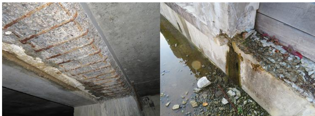
Figure 1 – Corrosion destruction of building structures.
